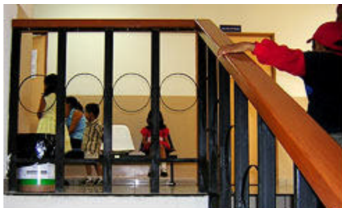
Lynn Underwood Flaws in U.S.-funded buildings in El Salvador include unsafe guardrails.
